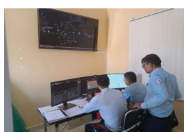
Electricity of Stung Treng
