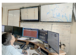
EDC - Dispatch Control Center (DCC)
